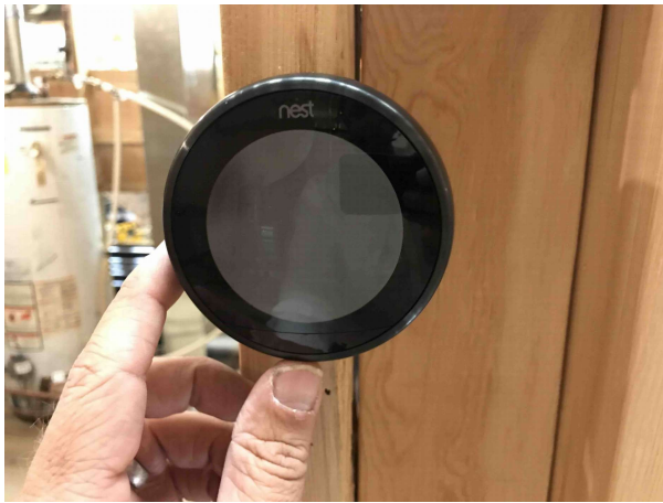
Image of a high-efficiency thermostat at the InterNACHI® House of Horrors® in Colorado.
